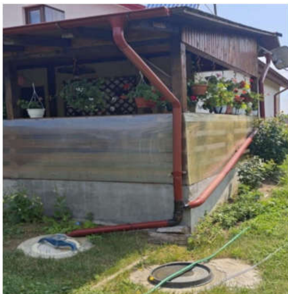
Figure 4: Improvised rainwater collection system. Source: personal archive.
